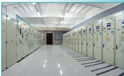
Electrical room of the "Leypysuo" DC traction substation 3.3 kV of the October Railway
