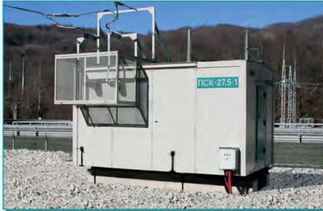
DC sectioning point PSK-25-1 (North Caucasus Railway)
