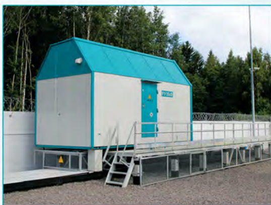
Medium voltage AC switchgear 35 kV module
