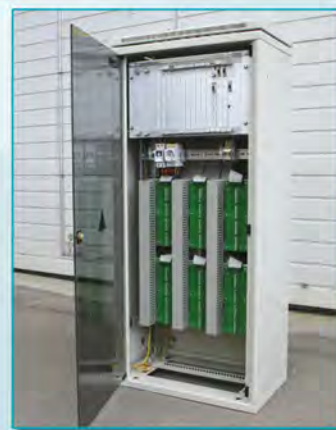
Telemechanical KP-B (TP) panel
