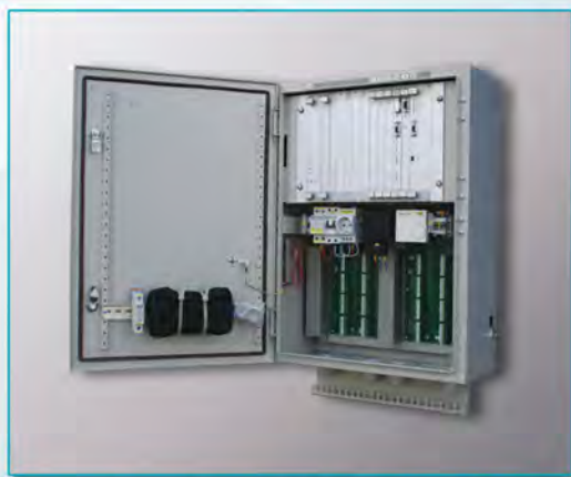
Telemechanical KP-M (PS) panel
