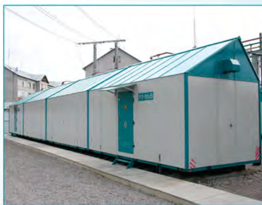
Medium voltage AC switchgear 6 (10) kV module
