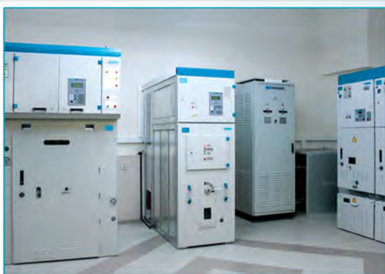
Simulation traction substation in Saint-Petersburg State Transport University
