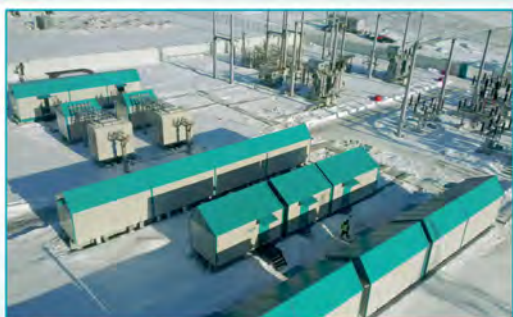
110/27.5/10/3.3 kV substation of Engels locomotive plant
