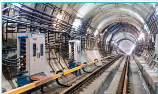
Traction network equipment 825 V of the Dostoevskaya – Mar'ina Roshcha section of the Moscow underground
