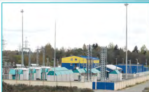
"Veymarn" DC traction substation 3.3 kV of the October Railway
