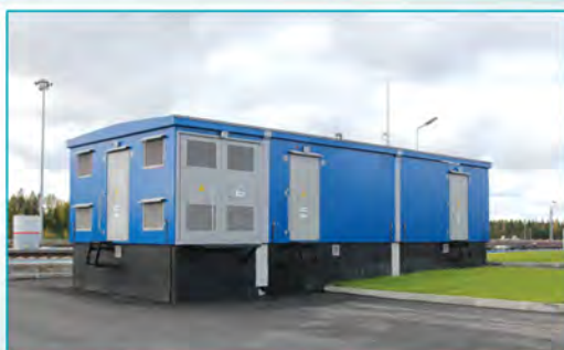
BKTPB modular package transformer substation in concrete shell at the Luzhskaya – Sortirivochnaya station
