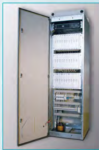
Disconnectors control panel
